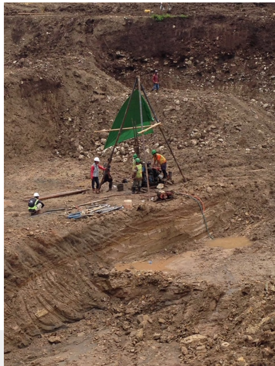
Figure 4. Rock cutting and drilling on the tuff siltstone mass of the outlet face at the Tanju tunnel.
