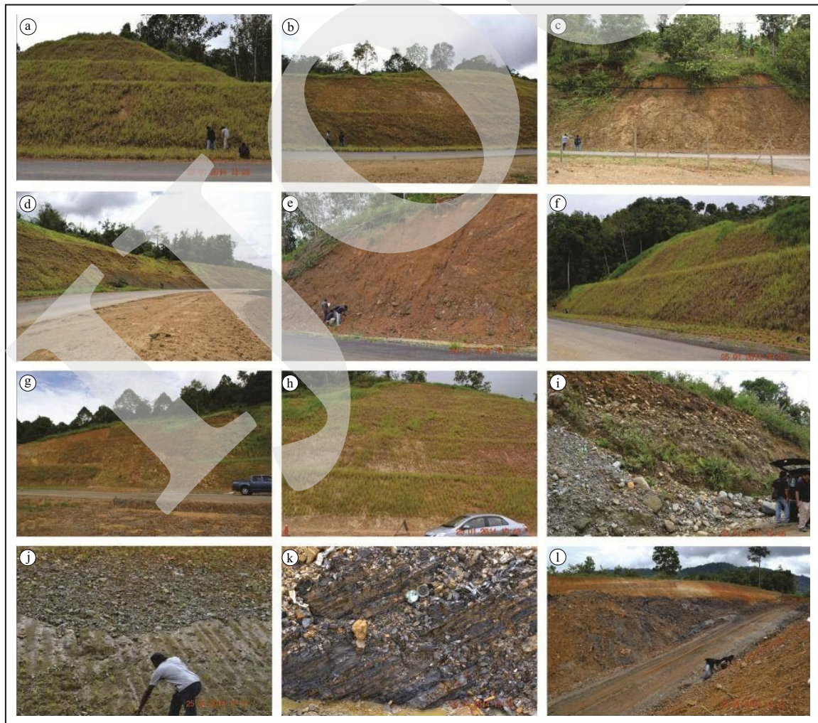
Figure 2. Slope sections. (a) slope 1; (b) slope 2; (c) slope 3; (d) slope 4; (e) slope 5; (f) slope 6; (g) slope 7; (h) slope 8; (i) slope 9; (j) slope 10; (k) slope 11 left; (l) slope 11 right.
