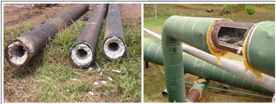
Figure 2. Amorphous silica scale on re-injection pipes (PT. Geodipa Energi, 2009).
