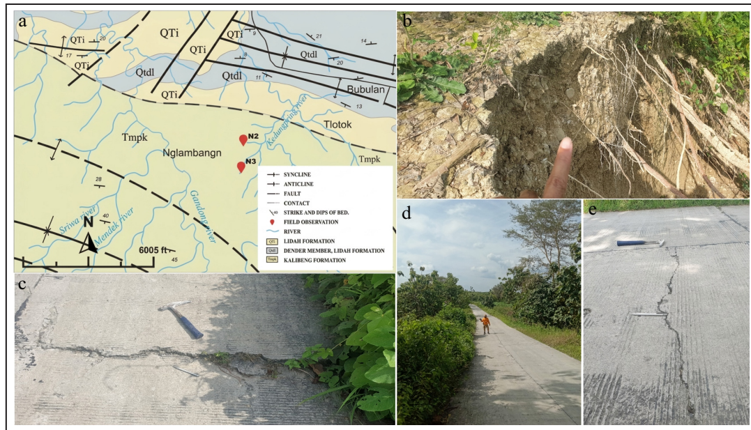
Figure 12. Manifestation of possible fault creep at N2 and N3 stations in the Nglambangan Village. N2 and N3 locations in The Bojonegoro Geological Map (Pringgoprawiro and Sukido, 2011) that close to the possible Kendeng Fault Zone (a), landslide at the N3 location (b), possible fault creep manifestation in N2 on the cemented road (s, d, and e).
