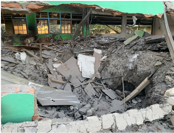
Figure 5. The impact of blast material of Lewotobi Laki-laki eruption on 3 rd November 2024, at 23:57 Central Indonesia Time on school building.
