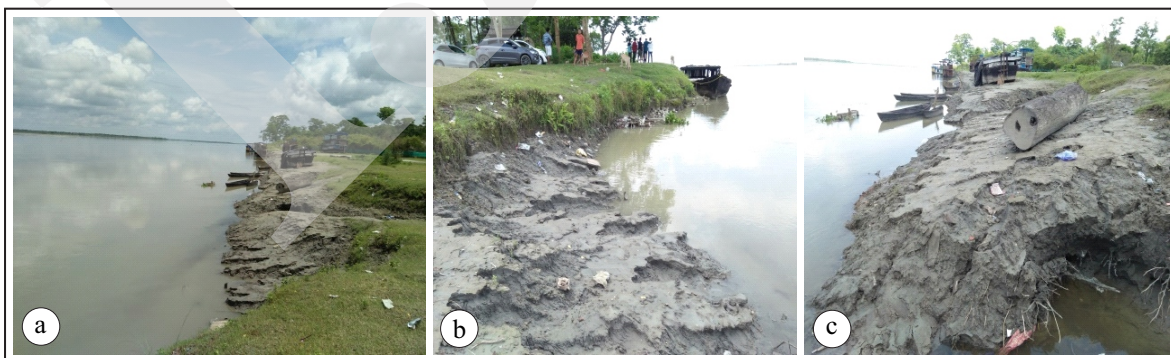
Figure 5. Photograph of bank erosion (Guijan Ghat).
